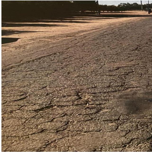
(Figure 1) Fox Road Pavement Deterioration
